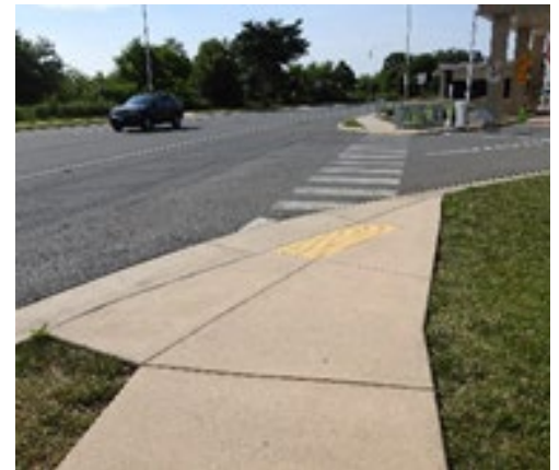
Noncompliant ABA Ramps and Crossing
