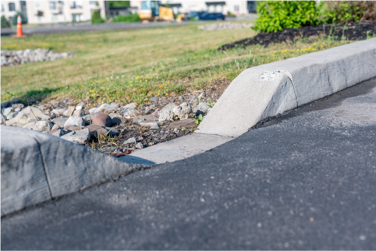
Swales Used to Transport Stormwater Runoff
