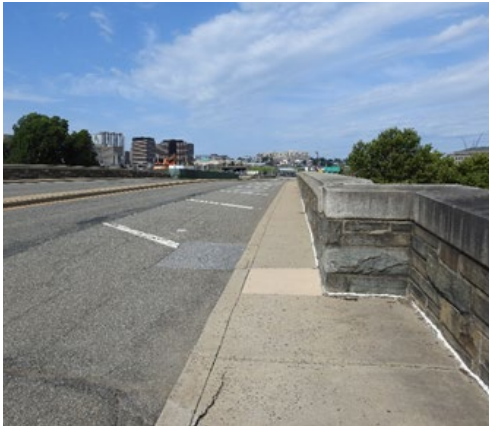
Substandard Sidewalk over Route 110 Bridge
