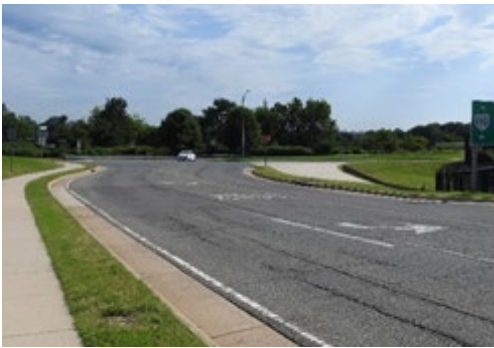
Deteriorating Pavement along Connector Road
