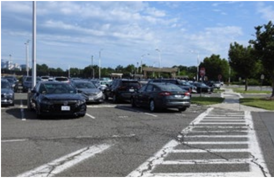
Rehabilitate Deteriorated Pavement in North Parking Lot
