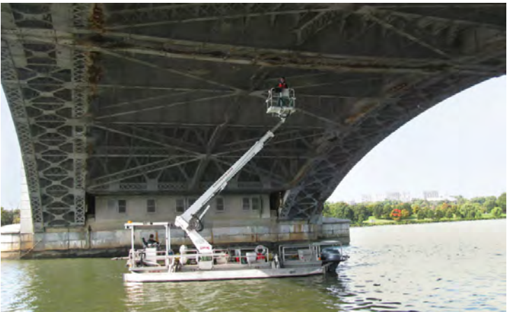
The existing bird nesting and dropping control system is installed at the entire underside of the bascule span along the underside of the existing trusses. The mesh density is 1" x 1" at a 45 degree angle hung using metal pipes. Existing bridge inspection methods involve removal of the bird netting to inspect the bridge elements from a boat lift.
