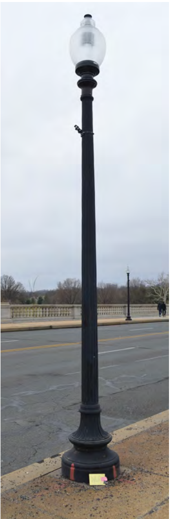
Cast iron lamp post
