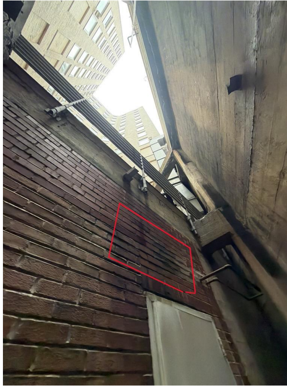
Figure 3 Boiler Intake and Flue Ducting Penetration Location at Bottom of the Air Shaft
