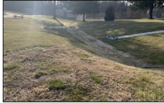
Grass stormwater swale with erosion control matting
