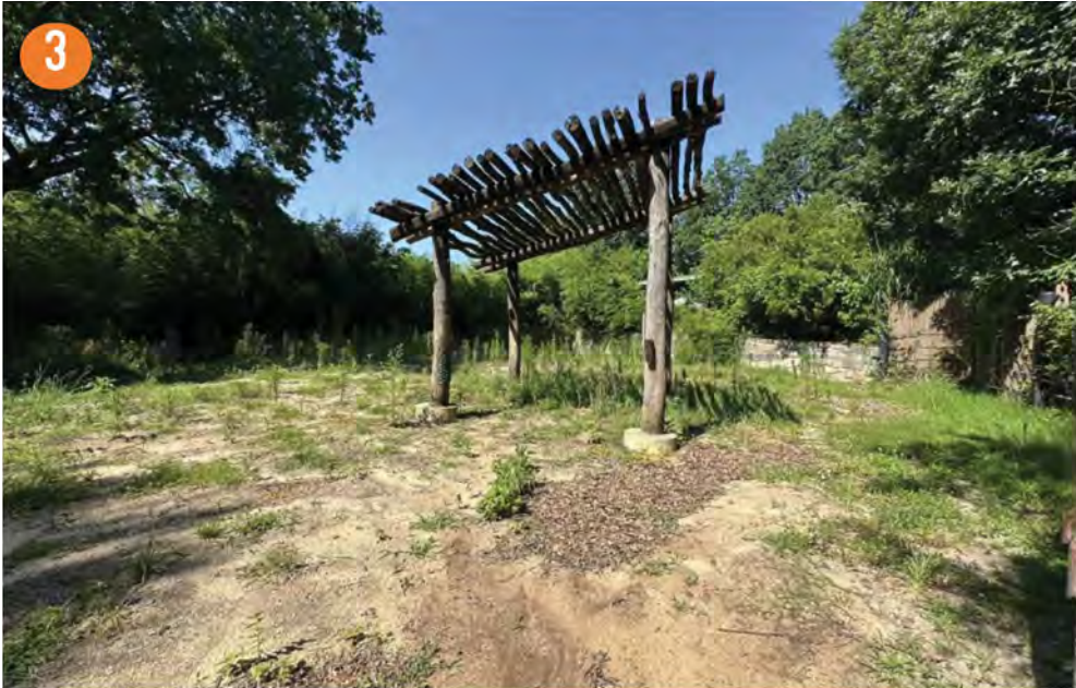
Bison Shade Structure
