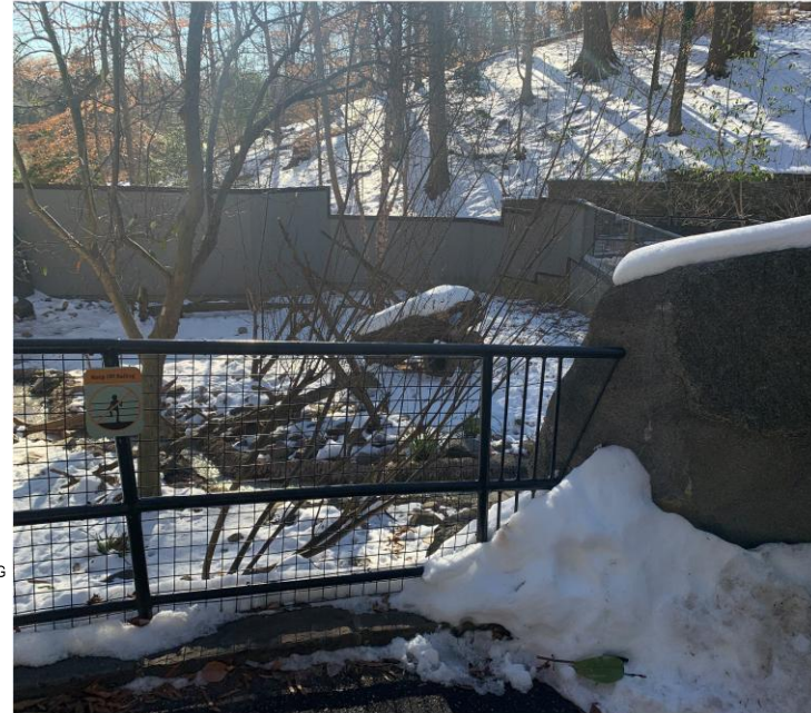
REFERENCE IMAGE FOR PROPOSED RAILING TYPE 1: Existing stone clad retaining wall with steel mesh netting guardrail at Otter
