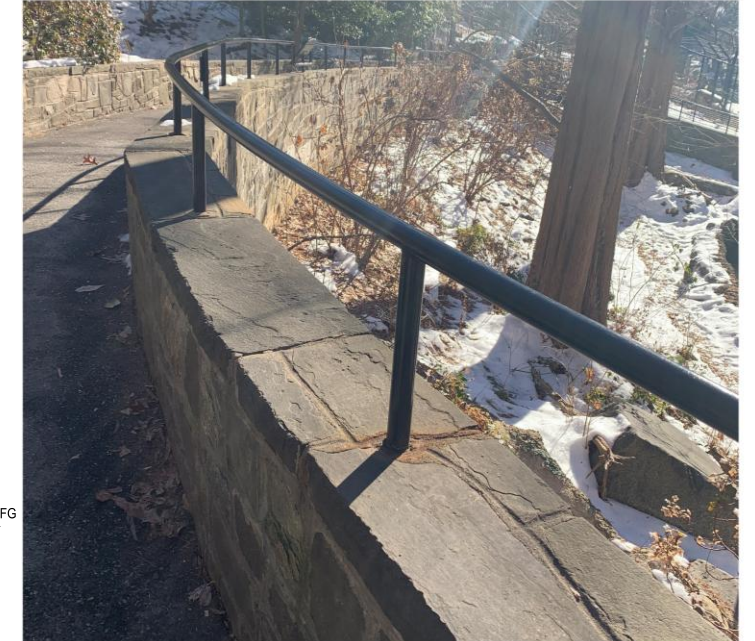
REFERENCE IMAGE FOR PROPOSED RAILING TYPE 2: Existing stone clad retaining wall with steel tube handrail at beaver
