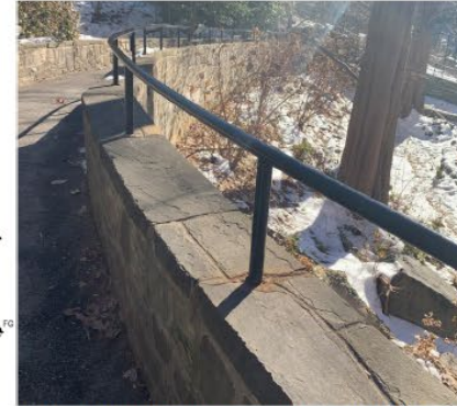
REFERENCE IMAGE FOR PROPOSED RAILING TYPE 2: Existing stone clad retaining wall with steel tube handrail at beaver
