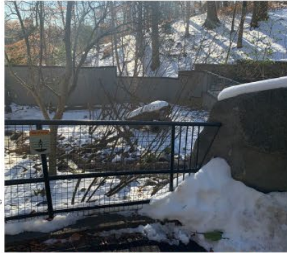
REFERENCE IMAGE FOR PROPOSED RAILING TYPE 1: Existing stone clad retaining wall with steel mesh netting guardrail at Otter
