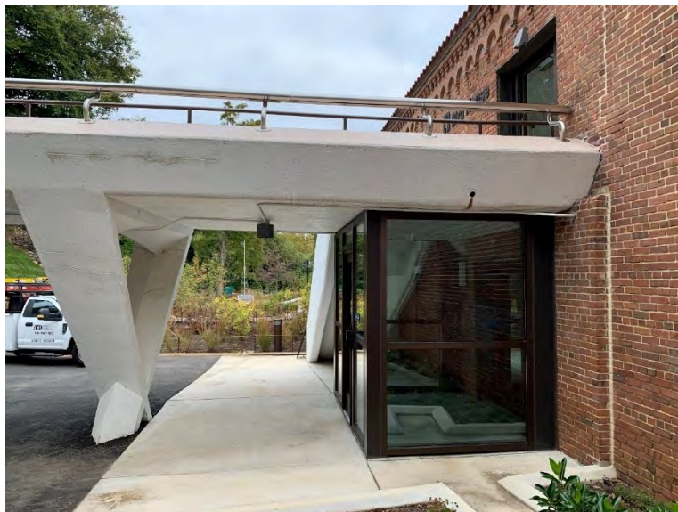
View from ground looking at intersection location of new walkway and existing GFA bridge
