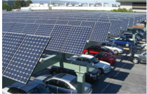
Solar panels in parking areas can provide shelter while generating energy.
