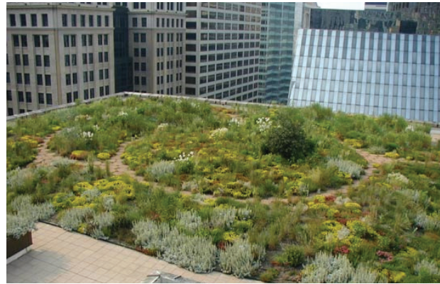
Green roofs can insulate the building as well as collect rainwater and reduce energy costs.
