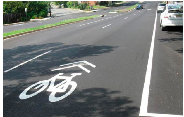
Share bicycle lanes will produce environmental benefits for the installation and health benefits for users
