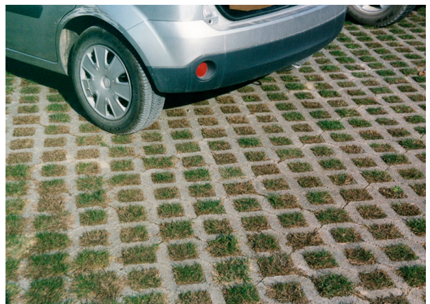
Porous pavement in parking areas will reduce the quantity of stormwater runoff
