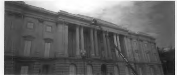
Figure 1. Low-to-medium-pressure steam (hot-pressurized water washing), is being used to clean the exterior of the U.S. Tariff Commission Building, the first marble building constructed in Washington, D.C., in 1859. This method was selected by an architectural conservator as the "gentlest means possible" to clean the marble. Steam can soften heavy soiling deposits such as those on the cornice and column capitals, and facilitate easy removal. Note how these deposits have been removed from the right side of the cornice which has already been cleaned.
