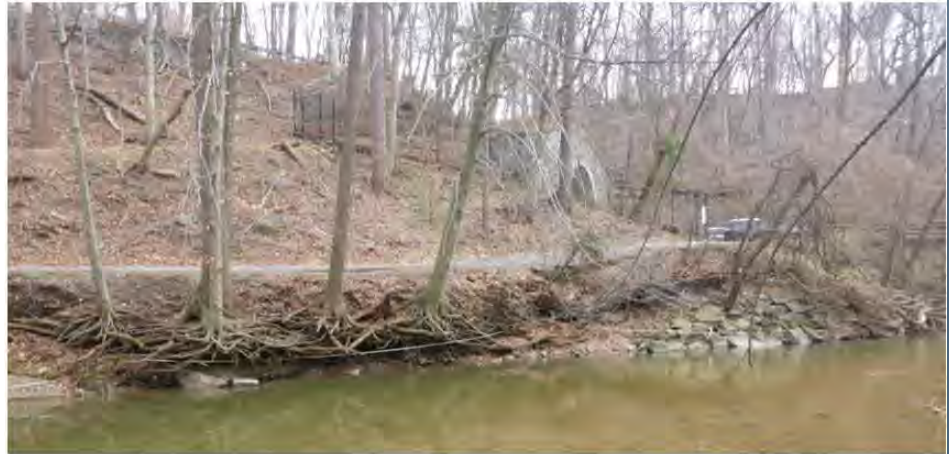
The northeast bank of Rock Creek in vicinity of the pedestrian bridge is eroding during heavy storms and undermining the existing trail.
